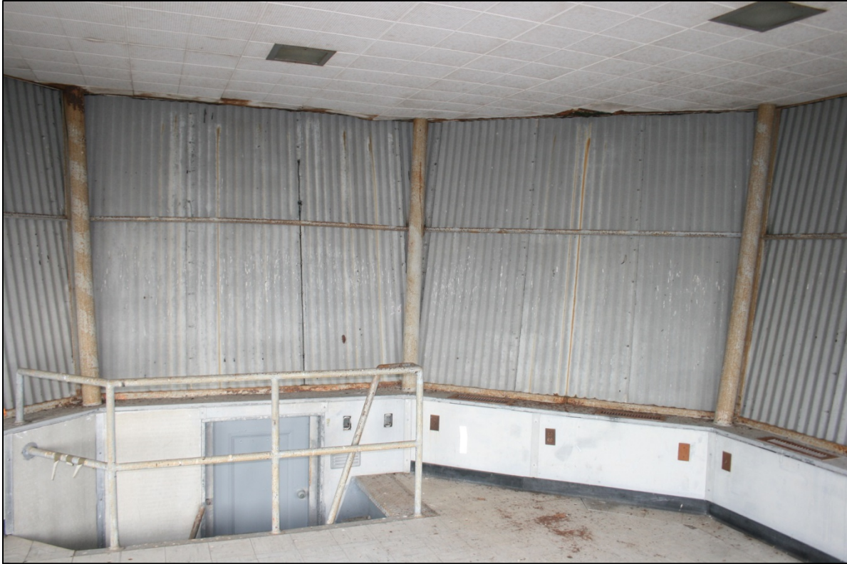
Figure 37: Building 1-14, control room detail view looking west
